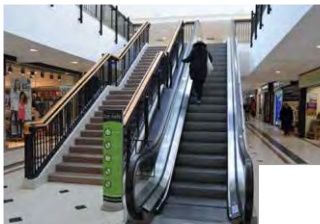
Lifts and Escalators
